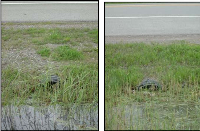
Photo 11 – View of the pipes that appear to connect the ditch east of the Rt 93 Bypass (left) with the ditch that is west of the Bypass (Right).
