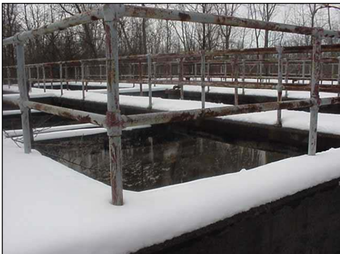
Photo 2 shows the Imhoff tank, which is a falling/drowning and possible explosive waste hazard.
