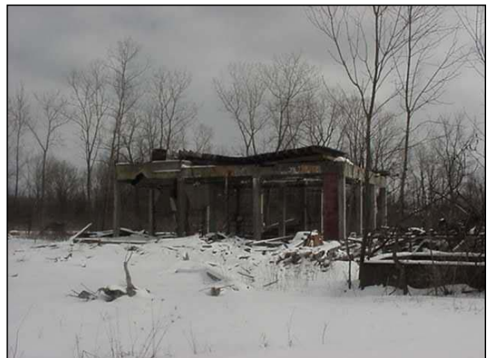
Photo 1 shows the Acid Neutralization Building that includes falling/drowning hazards, physical hazards due to structural instability, a possible explosive hazard, and friable asbestos.
