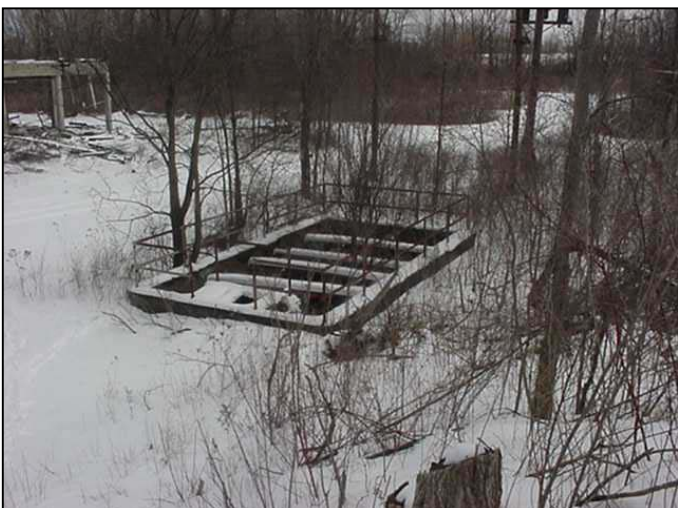
Photo 3 shows the chlorine tank, which is a falling/drowning and possible explosive waste hazard.
