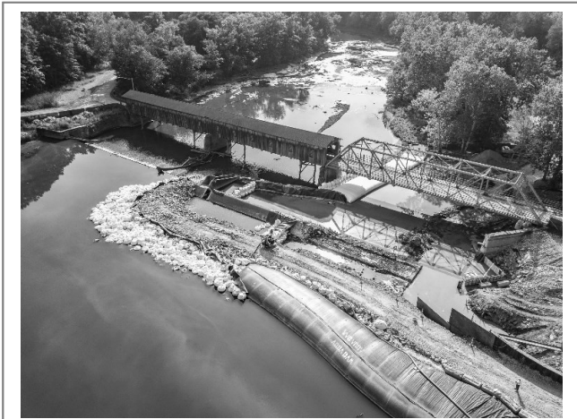
Figure 1 Drone photo of new dam during construction. The historic Harpersfield covered bridge is in the background.
