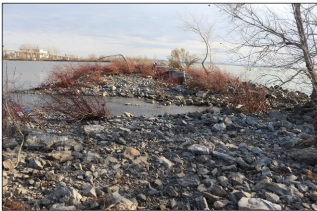
Figure 1: Close-up view of one of the breached areas of the break wall.
