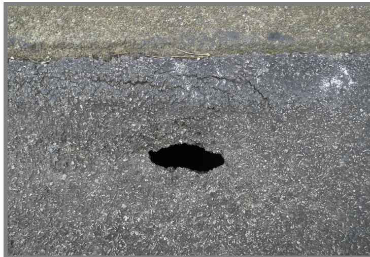
Existing Conditions — Sink Hole on Bike Path
