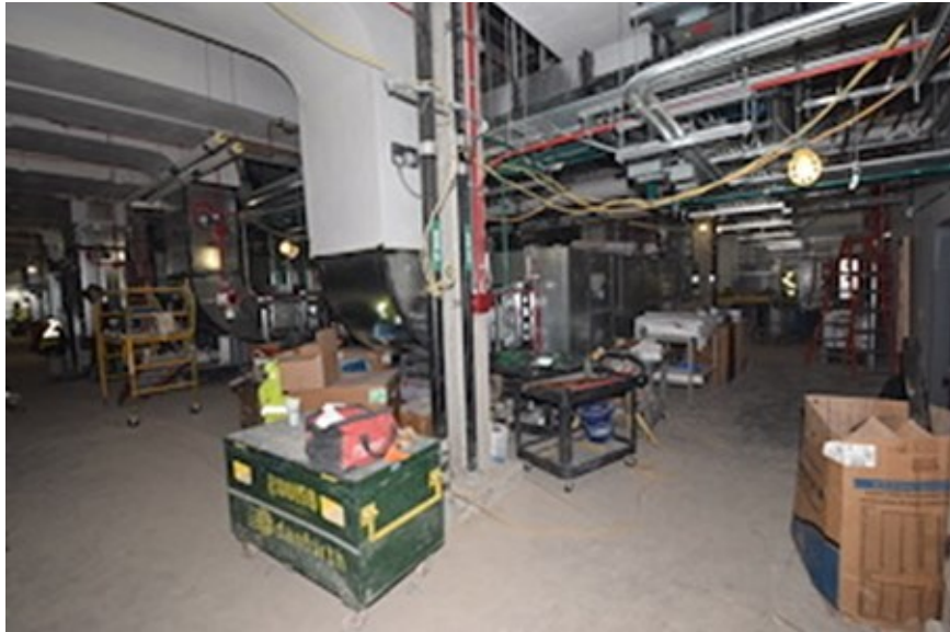
Bldg. 2 Mechanical Equip. Penthouse
