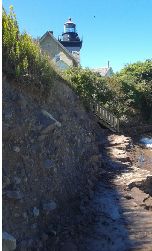
Significant shoreline erosion adjacent to the Lighthouse
