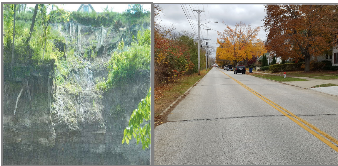
Slope failure looking up from Grand River (left) and view of Bank St. looking southeast (right)
