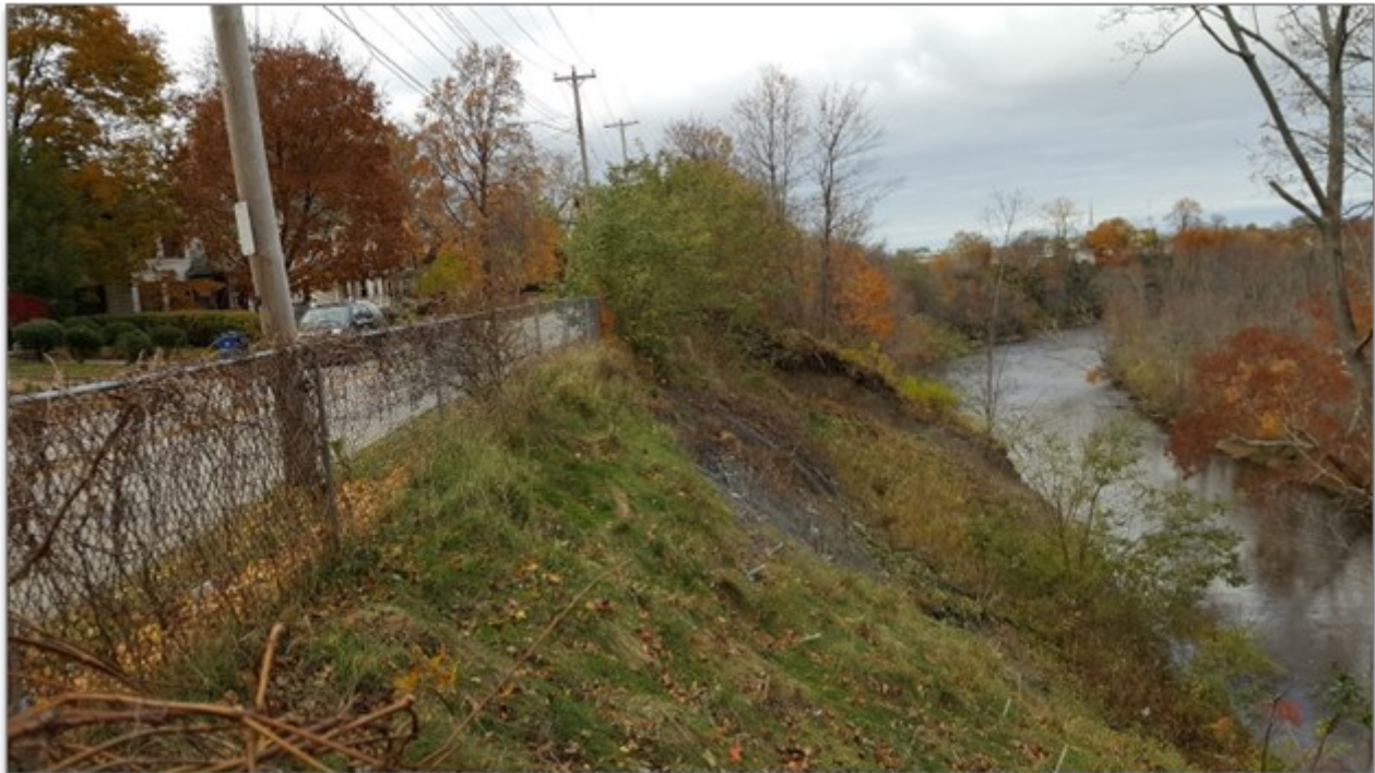
Side view of slope encroachment threatening Bank Street and utilities.
