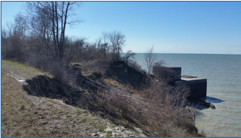
Photo 1 (April 2016) – Original road to the raw water pump station washed out with downed trees in background.
