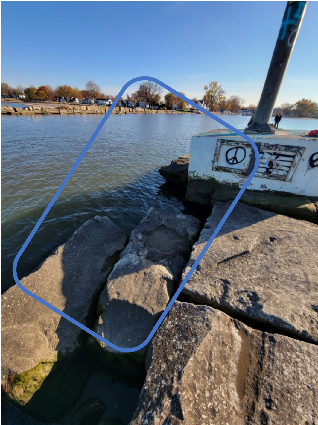
Photo November 2021 - significant stone loss
